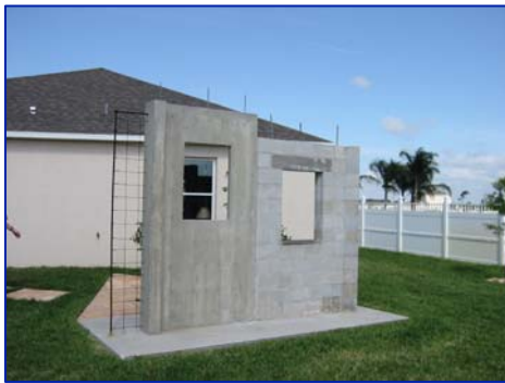
A mock-up of the Mercedes Homes cast-in-place concrete wall next to a standard CMU wall.
