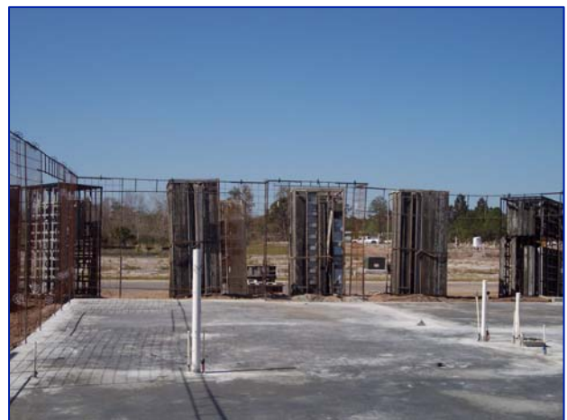
Mercedes Homes raises the reinforcing steel for their next cast-in-place concrete wall home. (Source: Mercedes Homes)
