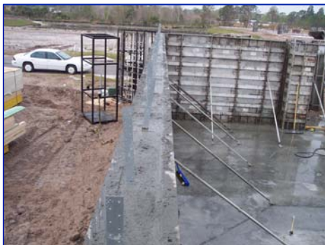
A cast-in-place concrete wall shortly after pouring and placement of truss tie-down embeds.
