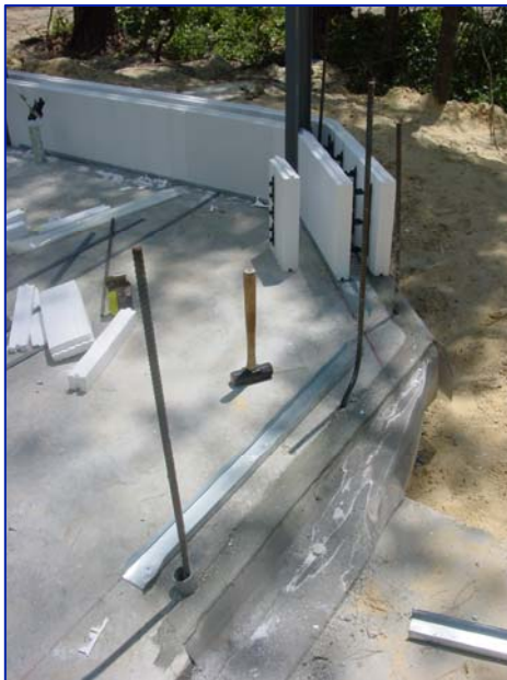
ECO-Block ICF wall being installed in the Madera Model embedded rebar. The Termimesh subsurface poison-free termite barrier is also visible.
