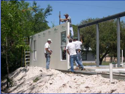
A four man crew can quickly and easily install the Home Front, Inc. SIP walls.
